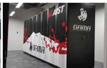
Server Room with GAMA
